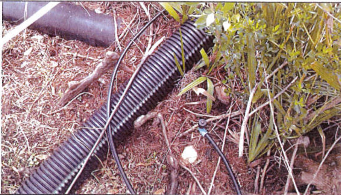
Photo 3: Exposed utility and irrigation pipes, northwest corner.
