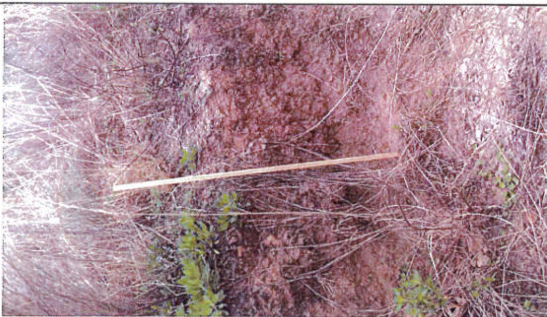
Photo 5: Slope toe erosion.
