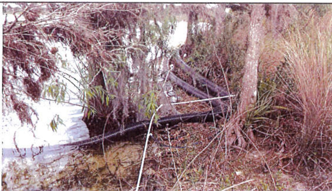
Photo 6: Exposed utilities due to slope erosion.
