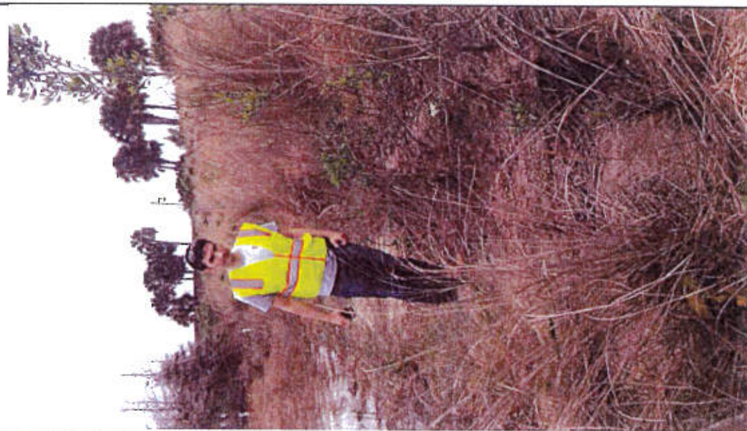
Photo 4: Slope toe erosion.
