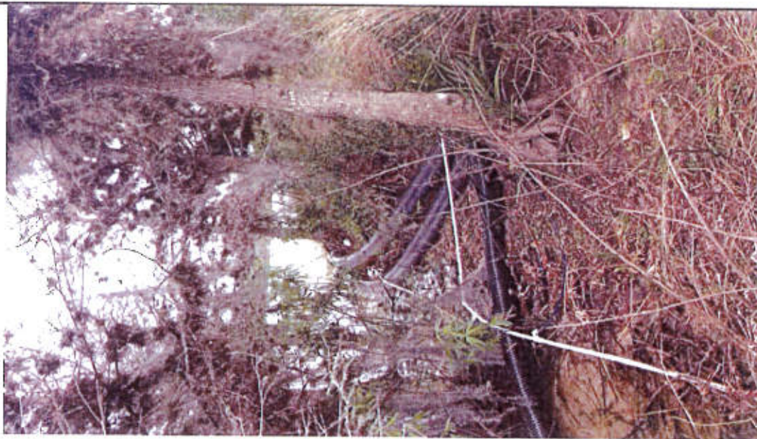
Photo 2: Exposed utility and irrigation pipes, northwest corner.
