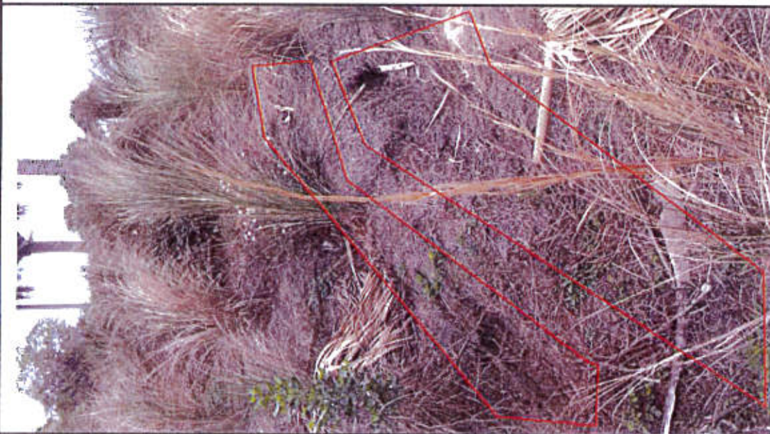
Photo 12: Slope erosion – northeast corner.
