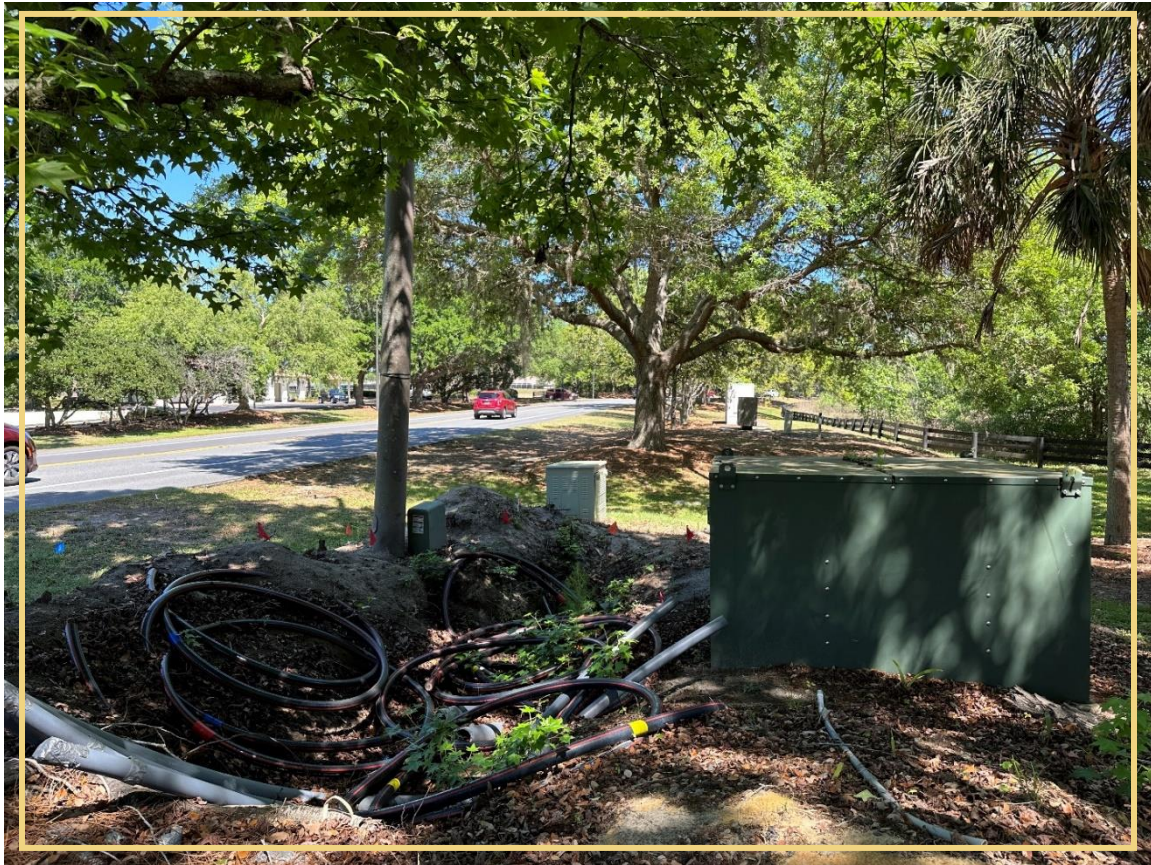
Photograph 7 – SECO Switchgear and utility installation
